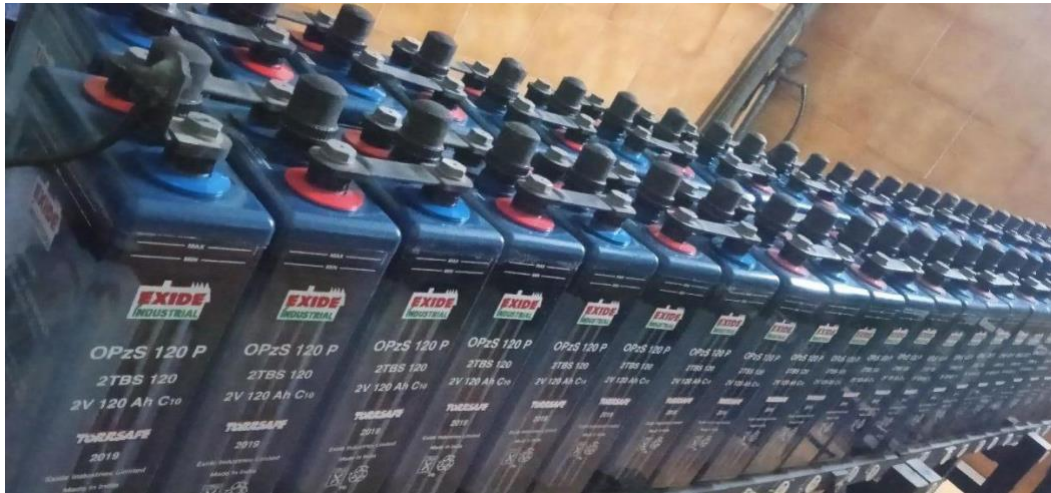
FIG.1.8:BATTERY BACKUP OF KOODALNAGAR SUBSTATION
